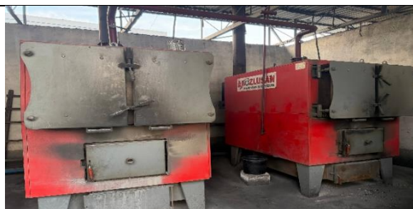
Clean Biomass System
