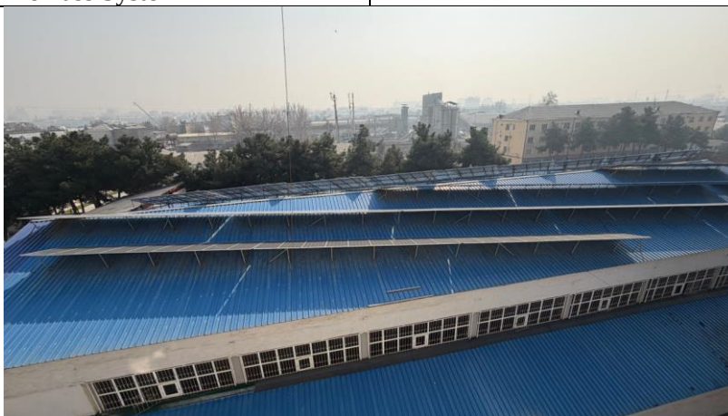
Roof and Façade Mounted Solar Panels
